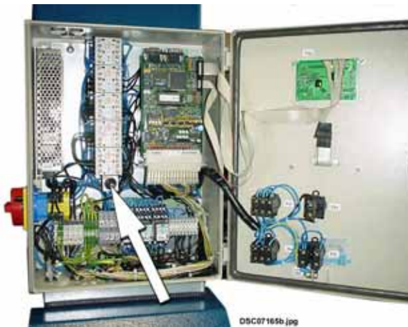
Pic 2: Position of the bypass switch
